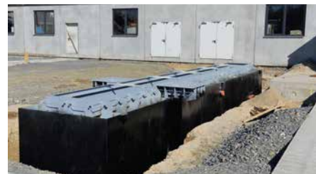
Once the concrete has set, the pit body can be cast in the floor.
