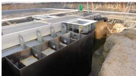
The double wall is now filled with concrete to achieve the required stability.
