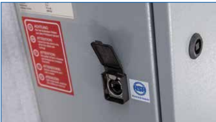
External data interface, e.g. for WiFi access point
